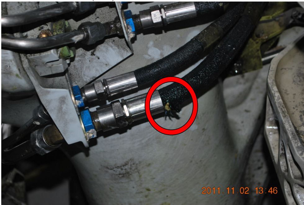
Photo 8. Damaged hydraulic hose of the right main landing gear of SP-LPC airplane.
